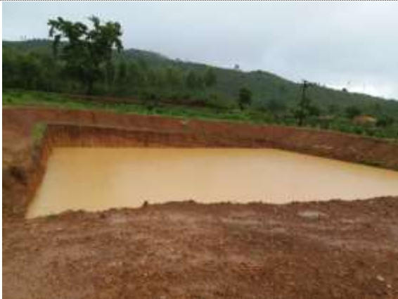
Rainwater harvesting structure constructed in 2016 (In rainy season)
