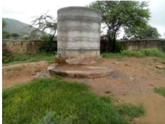
Existing drinking water facility in the school
