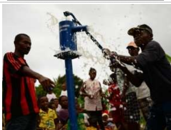
Installed hand pump
