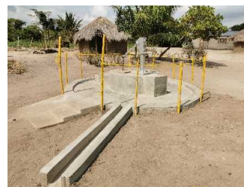
A completed well with a concrete platform that protects the groundwater source and helps maintain clean, safe water.
