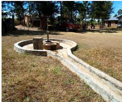
Non-functioning borehole well at Nyayo health center
