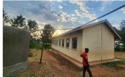
Gutters connected to the water harvest tank
