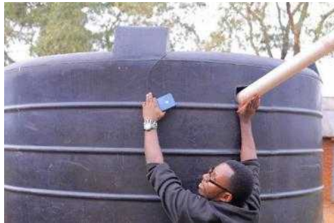
Damage to water harvesting tank
