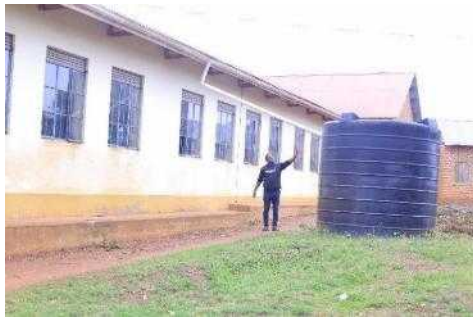
Damaged water harvesting tank
