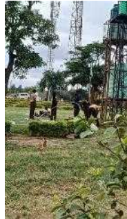
Connection of solar powered pump
