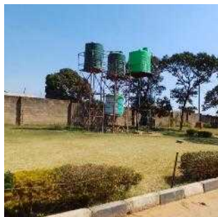
Water storage tanks supplied by an electric submersible water pump
