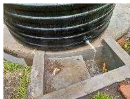
RWHS tank tap in service
