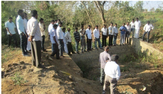
Before: Poorly maintained check dam
