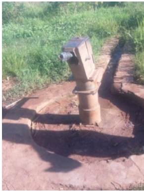
Before: A broken hand pump well
