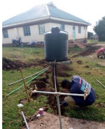
Connection of the tank and handwashing facility
