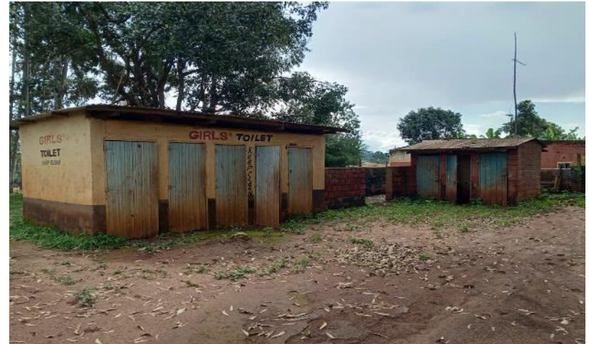
Existing latrines without hand-washing facility
